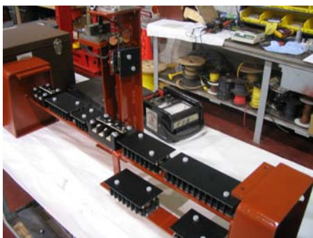
New Terminals and Wiring
